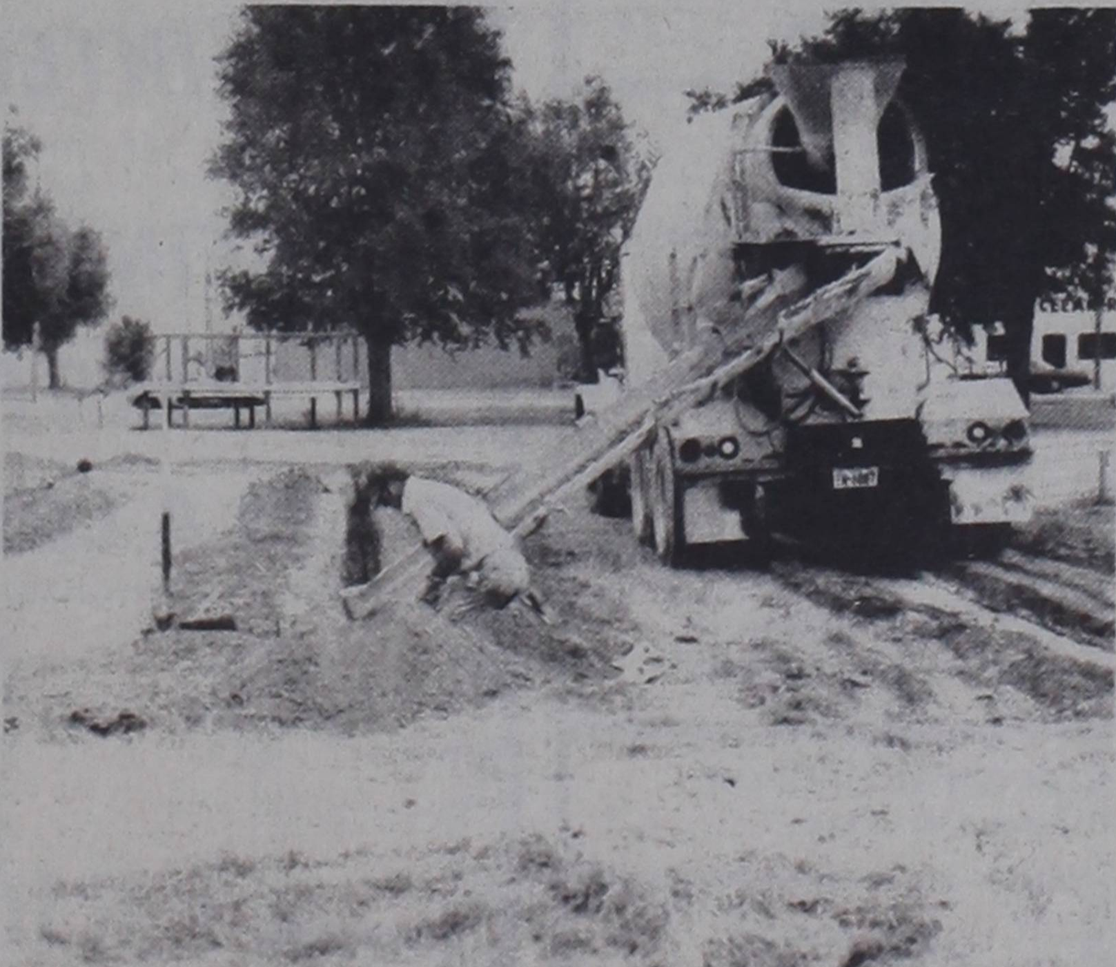
FOUNDATION POURED....Raymond Hamilton is shown as he is pouring the concrete foundation for the old Depot building. The Heritage Society has taken over ownership of the building.
