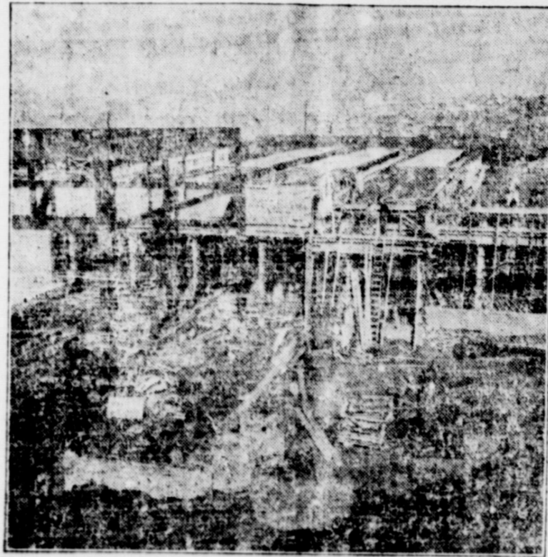
This photograph gives a realistic idea of how rapidly work is progressing on the Texas Centennial Exposition's huge lot in Dallas. All of the frameworks shown above are part of Livestock Building No. 2, one of two structures which will house the greatest stock show the United States has seen. The two buildings, their construction cost close to $100,000, will contain an ultra-modern veterinarian hospital.
