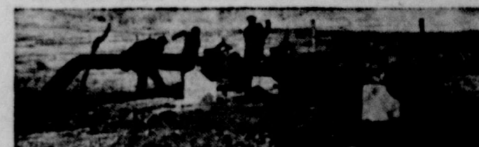
BEHIND GAS SERVICE there is something to build, paint, or repair every day, oftentimes in remote places. Above, a crew completes a control valve installation, part of a new compressor station. In the last three years, Lone Star has invested over $100 per customer to assure dependable service. Yet, you enjoy convenience and comforts of natural gas service for a year around average of less than 15c a day.
