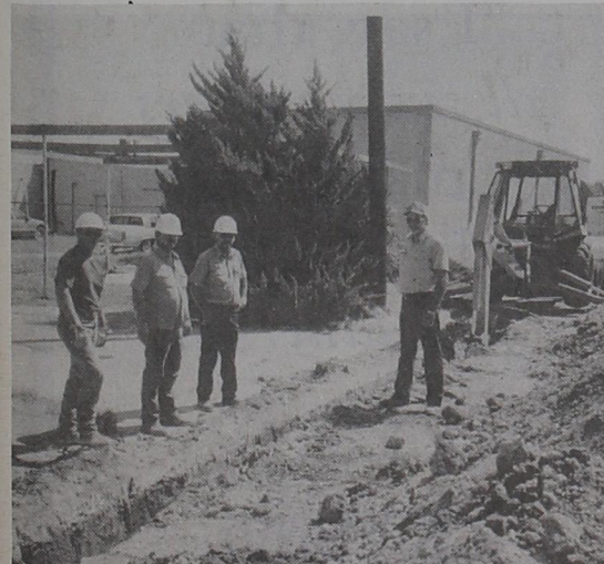
RE-ROUTING WATER.....City employees are shown on 6th Street, relaying water pipes that will eventually replace all water lines on Main Street. By next year, there will no longer be water pipes on Main Street as TX/DOT plans to re-do Main Street beginning about the first of the summer in 1997.
