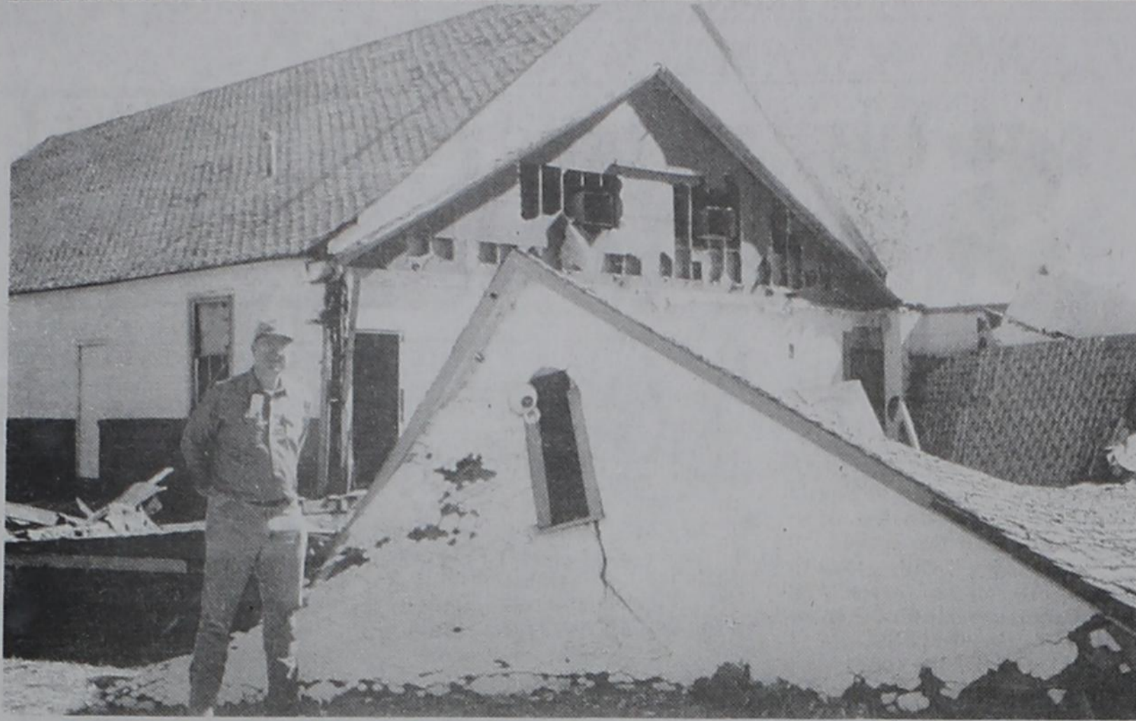
PREACHER BRINGS THE HOUSE DOWN.... Reverend Alvin Petty, pastor at Calvary Baptist Church is shown with the remains of the back part of the old sanctuary which was torn down last week. The church is remodeling the old sanctuary into a fellowship hall. ron carr photo
