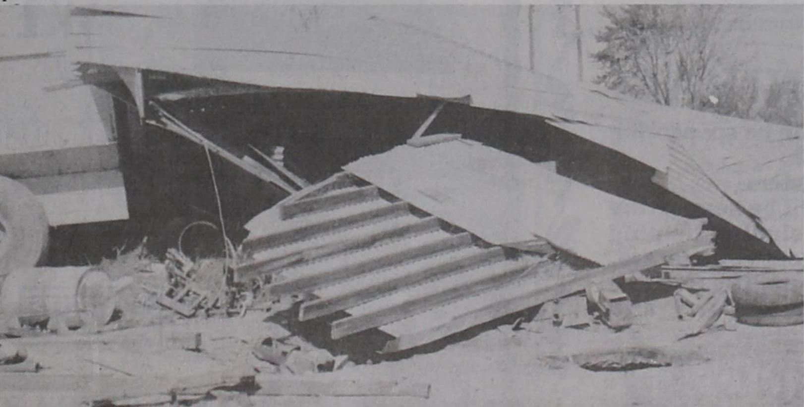
STORM DAMAGE.... The quonset barn belonging to Johnny Hand was destroyed by the August 27 storm. The barn, located east of Hub on Highway 86, was leveled by the storm, and came down on top of its contents.
