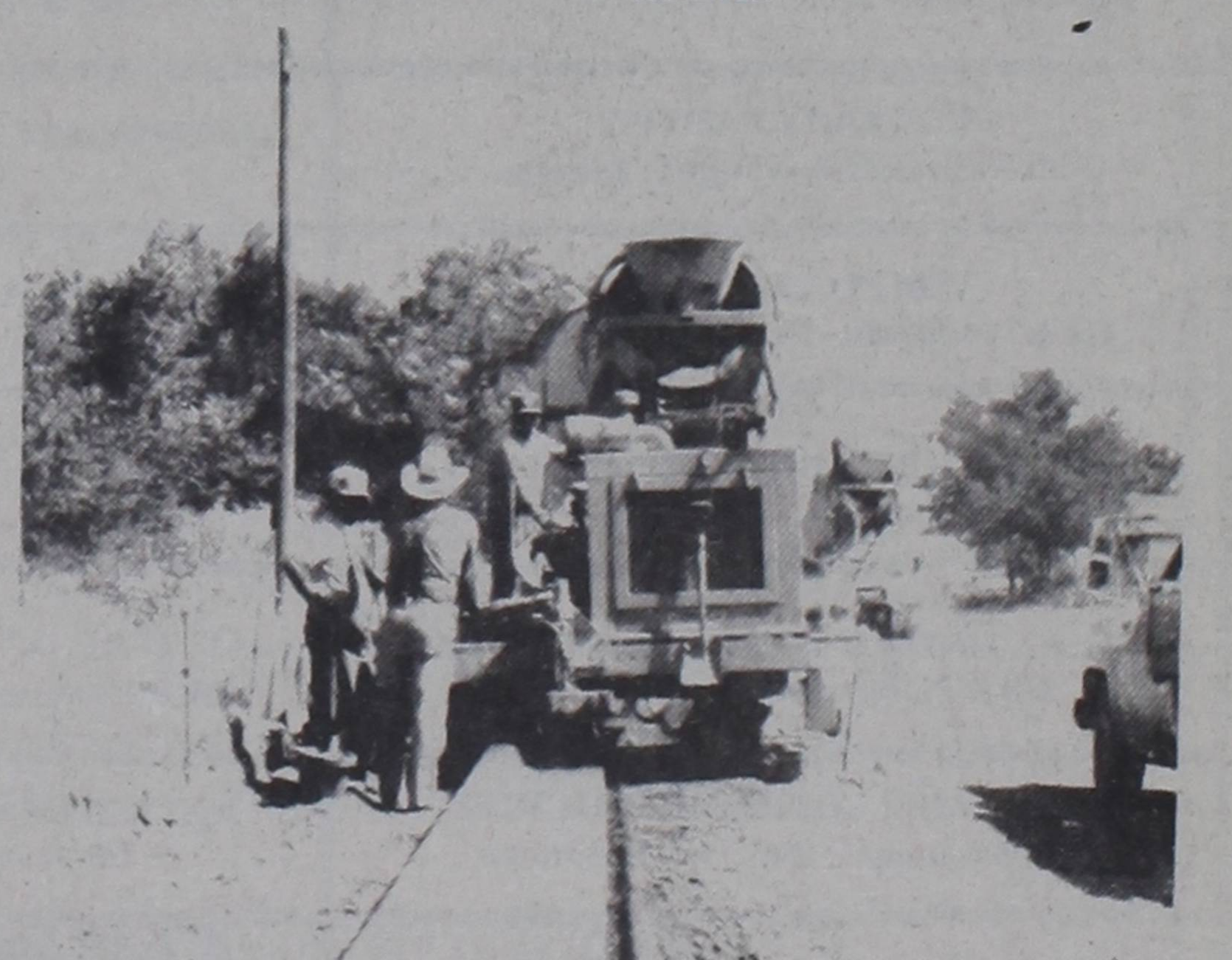
CURBS GO IN...A new method of laying street curbs is being used by the Applan Corp., at the paving project in Friona. The curbs were being installed on Thursday on Prospect Street. Rather than using forms, as has been the case for years, the curbs are molded by a machine, shown.
