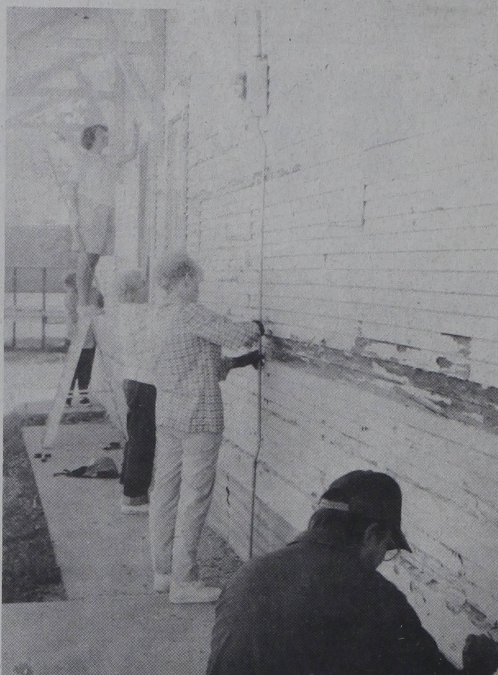
DEPOT WORK.... The faithful few who turned out for a work day at the depot last Sunday are shown scraping the paint off the exterior of the building to get it ready for repainting. A second work day is scheduled this Sunday, October 4.
