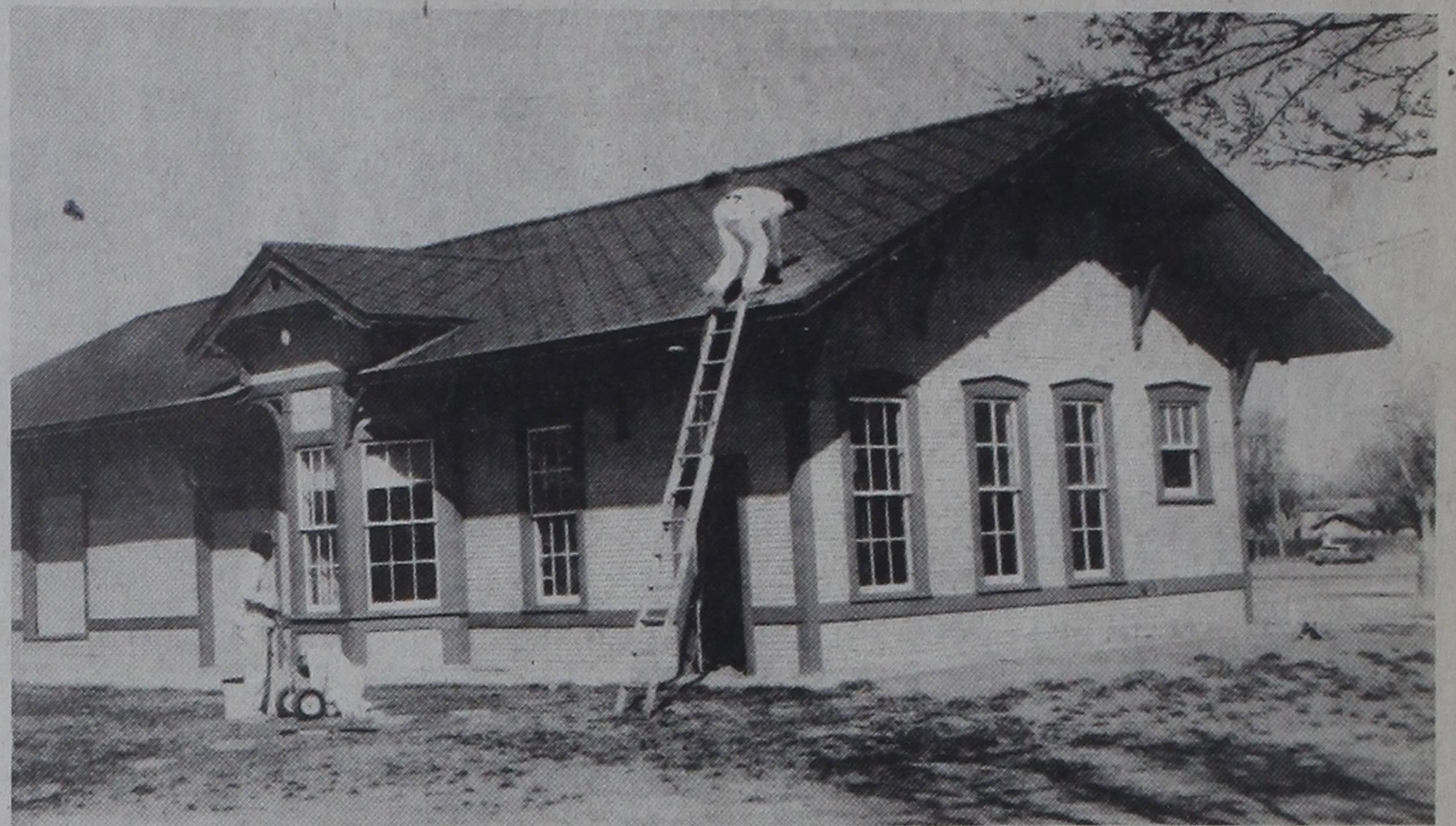
PAINT JOB FINISHED...Larry and Julio Pesina of Hereford are shown putting the finishing touches on the new paint job on the old Santa Fe Depot, now located at the City Park. The Heritage Society is soliciting donations to help with the renovation and improvements to the depot.
