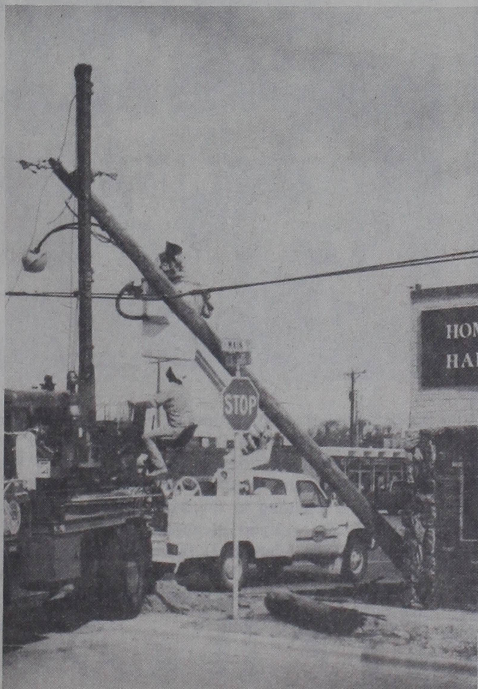
POLE PROBLEM... The power pole which also serves to hold the street light at 10th and Main, was severed earlier this week when a large truck turned the corner too sharply. A crew from Southwestern Public Service Company is shown making the repair.
