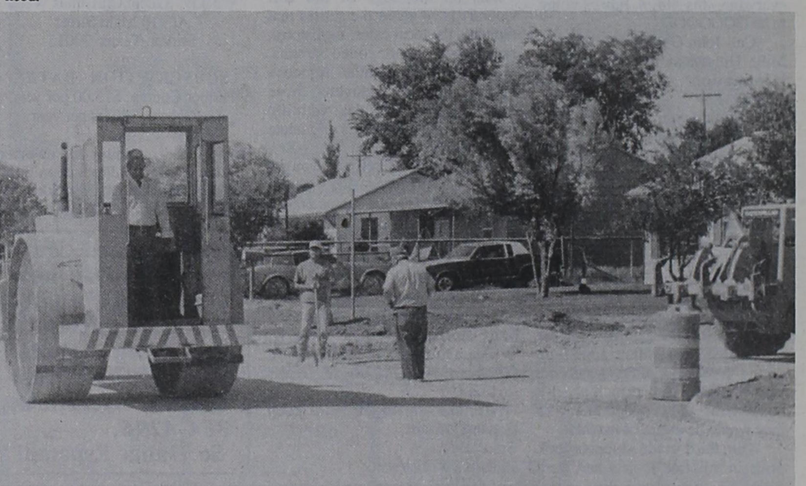
STREET PAVING... A crew from Amarillo Road Co is shown getting a couple of blocks on Walnut Street south of Highway 60 ready to pave. This is part of the five blocks of new paving received by the city through a state grant.
