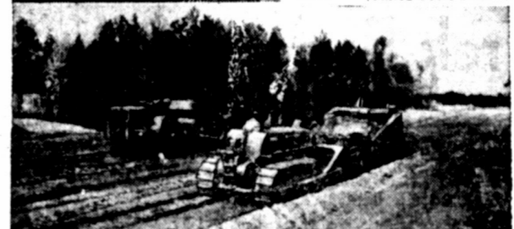
ROADS FOR TRANSPORTATION —Earthmoving equipment such as these International Harvester giants are very necessary to most forms of transportation. Before sleek automobiles and streamlined buses can skim over the ribbons of concrete and asphalt, high-speed earthmovers and crawler-type tractors, must first make the roadbeds. Fleets of equipment similar to these units, move millions of yards of rock and dirt in incredibly short spans of time and at surprisingly low costs.
