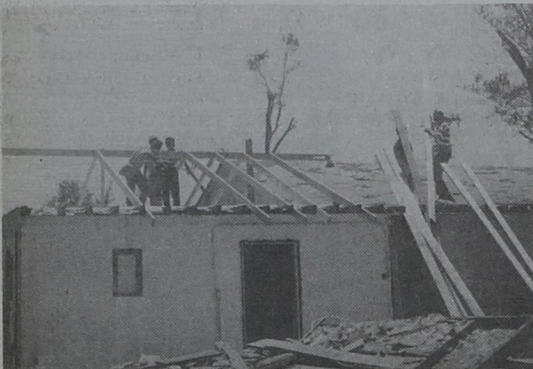
BI-PRODUCTS REBUILDS --Workmen reconstruct the housing and plant at Bi-Products on So. 214
