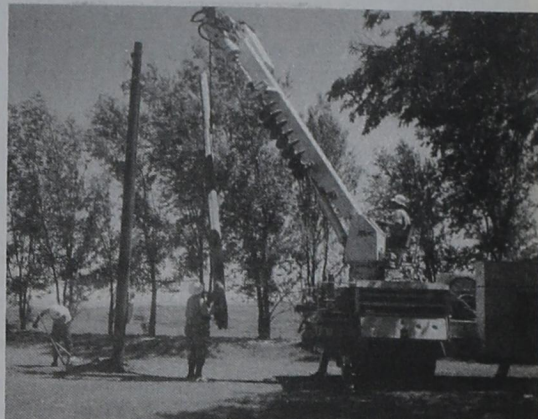
UTILITY WORK--SPS and REC workers were busy as beavers around Friona last week as they repaired poles, worked on lines and restored services to the citizens of this area. Top photo shows SPS working in area of Highway 2397 south of town. Lower photo shows REC putting in a new pole on the Doyle Cummings place west of town.
