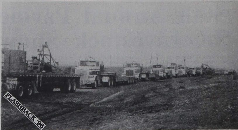
WIDE LOADS..... This convoy of wide horsepower was used to bring the huge track moving cranes in last week as work continues on the Santa Fe Railroad construction.
