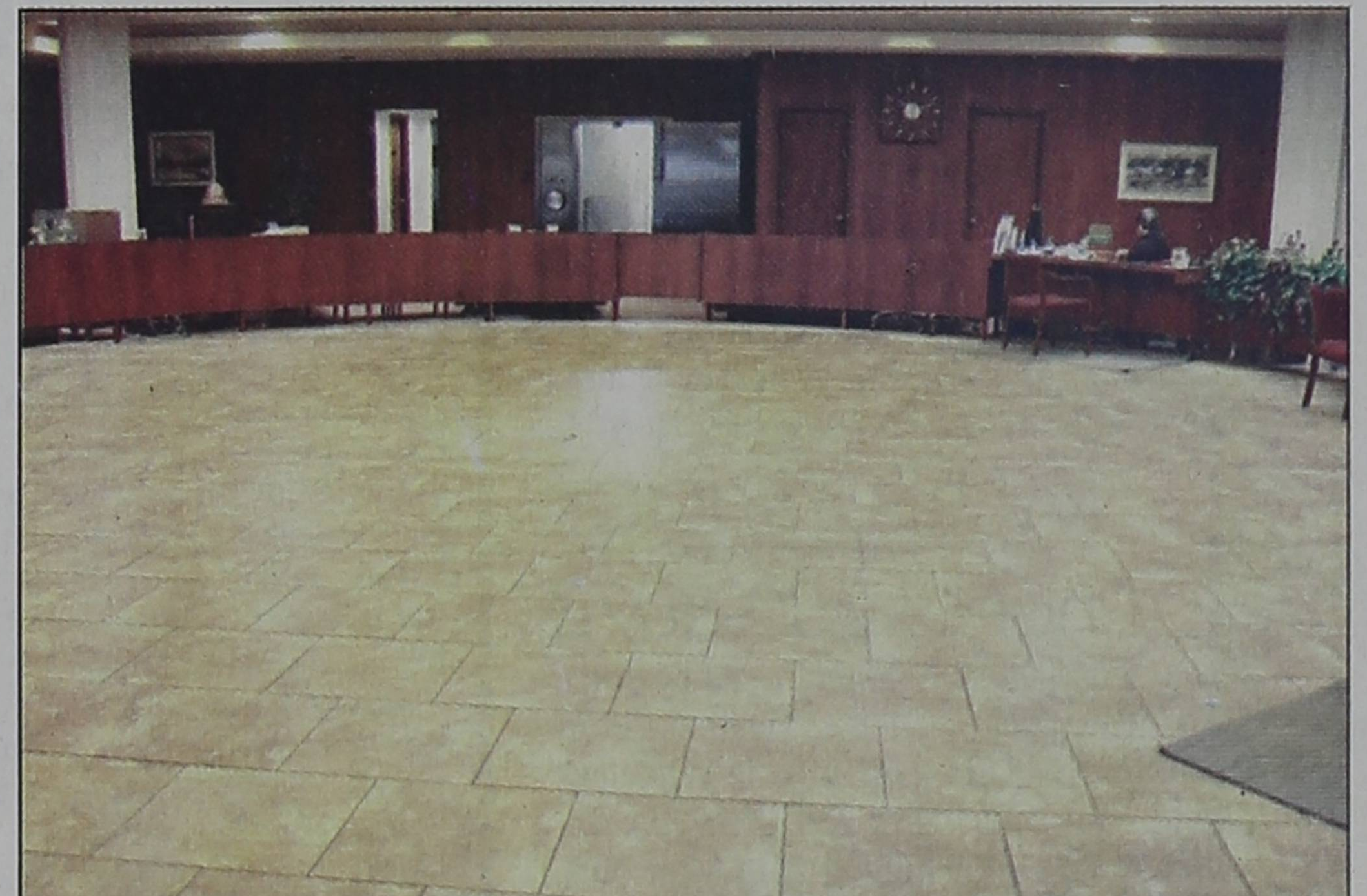
The lobby of Friona State Bank is getting a new look. The familiar tree and seating in the middle has been moved out to make way for new flooring. The kitchen, break room, and community room also have new flooring. New carpet is planned for the area behind the tellers and in the private offices.
