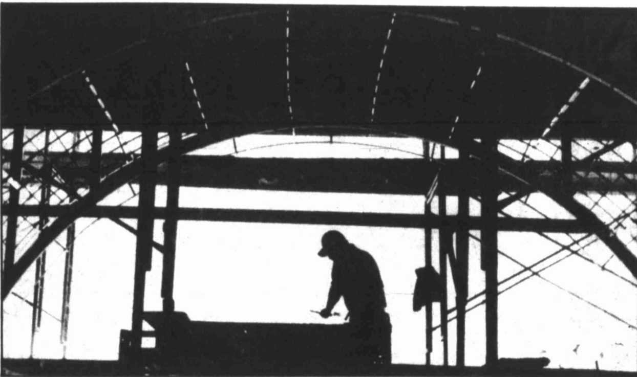
David Askew adds metal lathing to an arch in the new wing of the Heritage Museum in this October 1990 file photo. The new addition to the museum will be unveiled April 4.
