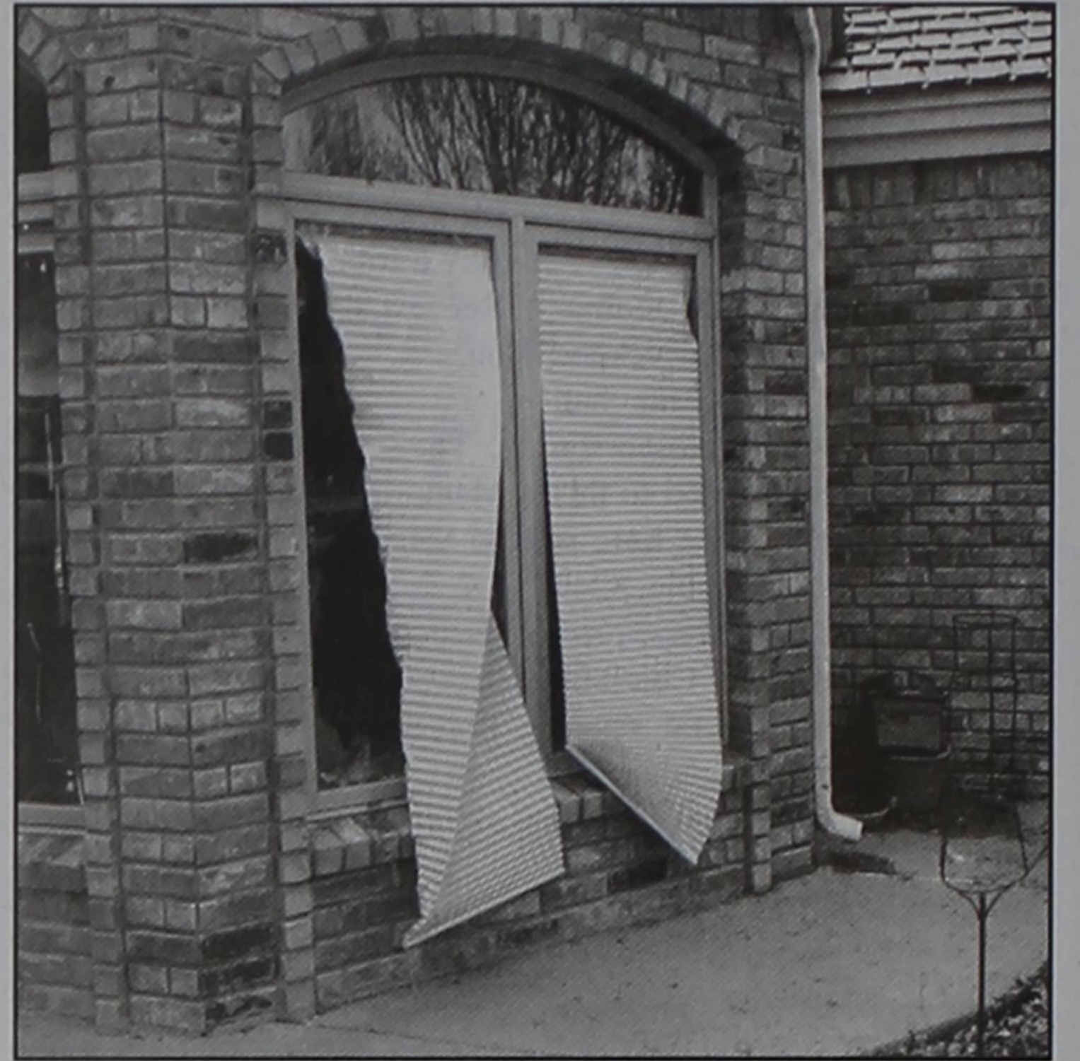
Hail damage in the western addition.
