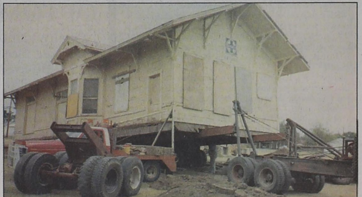
DEPOT ON THE MOVE...In August 1986, Levellen Construction Co., took on the massive job of moving the old Santa Fe Depot building from its original home, beside the railroad tracks, into the City Park. This coming Sunday, Friona will "Celebrate The Depot" in the Park on the 20 th anniversary of the Community Heritage Society. This charitable group was formed to oversee the moving, renovation, and upkeep of the Depot.
