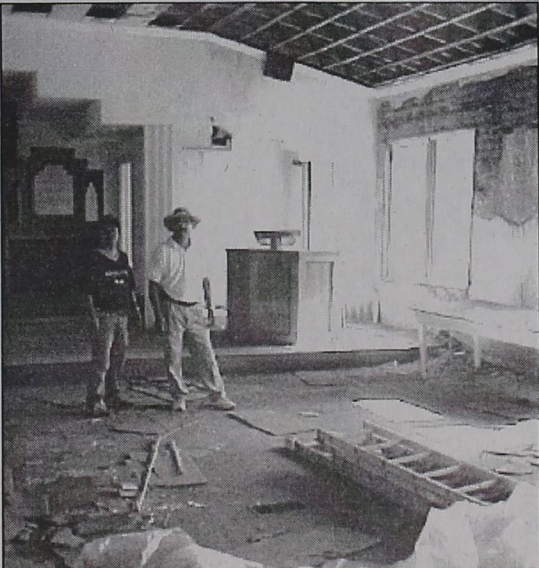
THE PARMER COUNTY Heritage Museum is progressing slowly. Billy Cantu, left, and Wally Castillo of Hereford Pre-Plastering & Painting are shown inside the top floor of the former Congregational Church. They are sealing windows and preparing to paint the interior.
