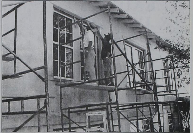
SCAFFOLDING IS UP around the old Congregational Church which is being rebuilt to house the Parmer County Heritage Museum. Above, Wally Castillo and Billy Cantu of Hereford Pro-Plastering & Painting are sealing the new windows before painting and remodeling the interior. ron carr photo
