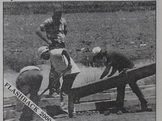
WORKERS FROM Ruben's A-1 Construction of Lubbock are installing the parking lot concrete curbing at Prairie Acres Heritage Estates. Shannon Cochran and Jeff Williams of T&S Concrete in Friona are shown delivering another load of concrete at the construction site. ron carr photo
