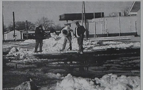
WORKERS are shown clearing a portion of Euclid Street near the junior high school as school was set to resume this week.
