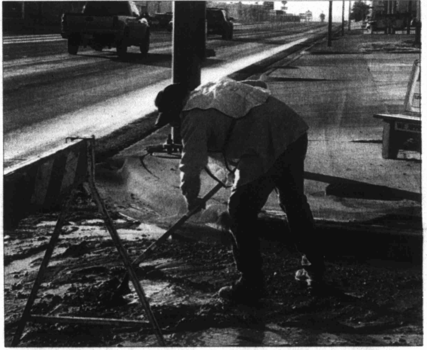
Ray Bryant, an employee with the city of Big Spring Water Department, works to repair a broken water line at the intersection of 18th and Gregg Street early this morning. More than 50 main water line breaks have been reported in the city since freezing weather gripped the Crossroads area.
