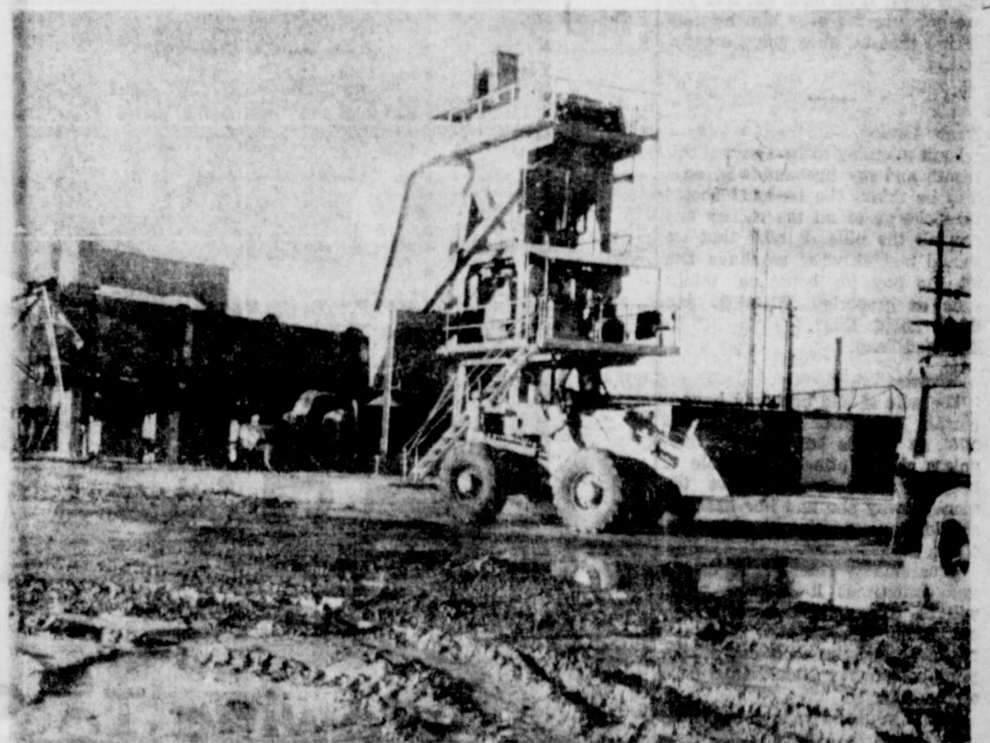
—We operate our own asphalt plant on Waco Drive near Brazos
