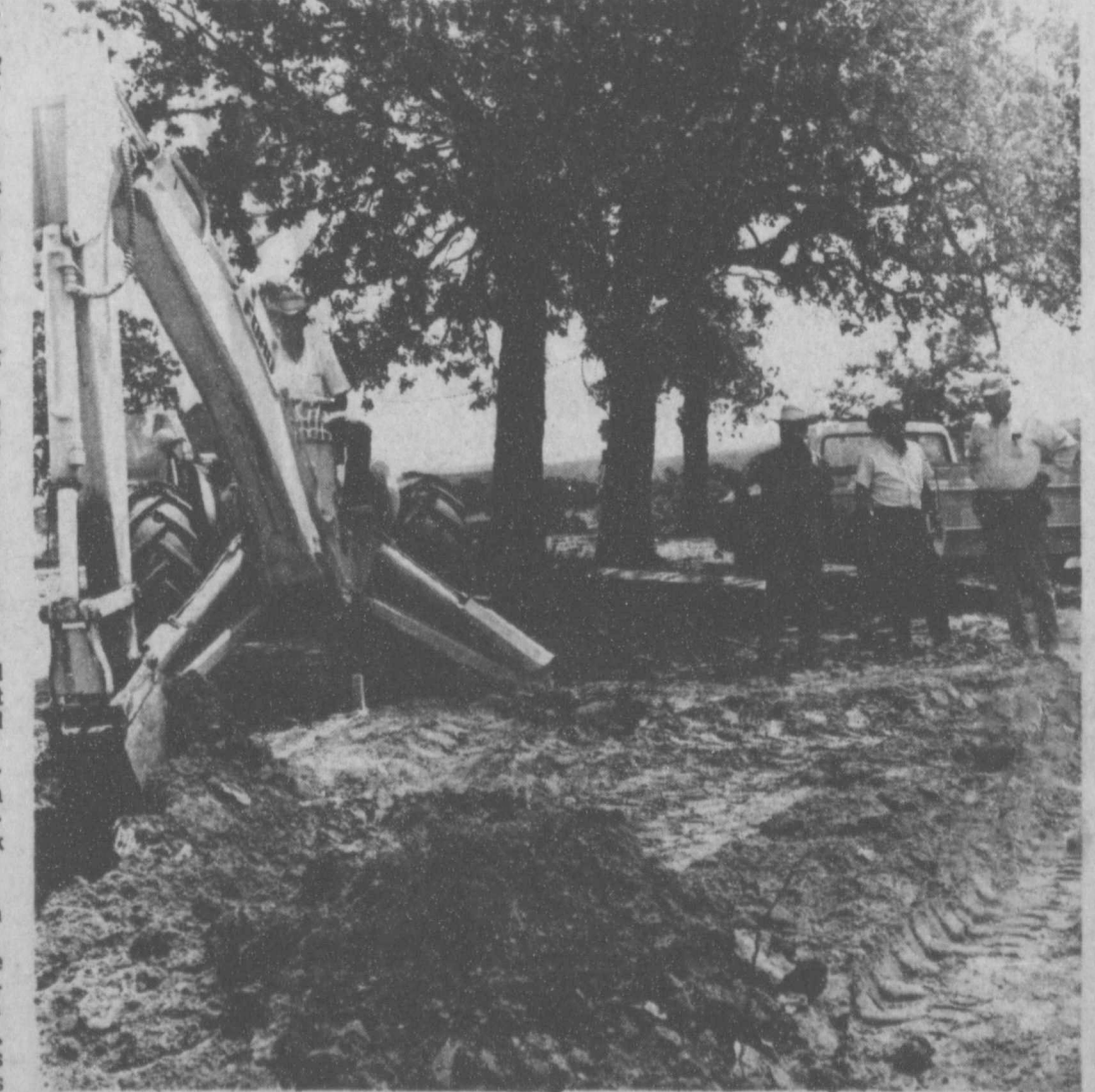
Construction work at L. T. C. Corporation began this week as Billy Pollard and Dixon Lumber Co. broke ground for the foundation of the clubhouse. The $100,000 clubhouse and cottage facilities will be completed by late July. L. T. C. stockholder, Homero Blancas played his way to $25,000 in the Colonial National Invitation.
