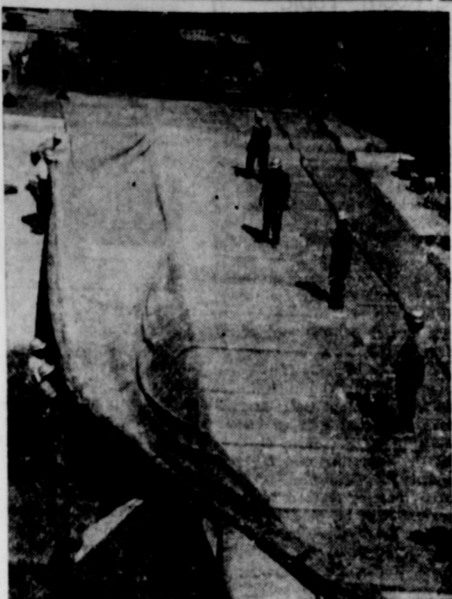
ROLLING OUT THE CARPET —Sixty feet below the surface of the ground in downtown Houston, workers stretch out a Butyl rubber carpet on which the 44-story Humble Oil & Refining Company building will stand when completed in 1962. The Butyl membrane will set as a water barrier for the foundation of the building. This is a unique application of the durable, flexible synthetic which is produced at Humble's Baytown Refinery and is widely used in everything from hot water bottles to conveyor belts, tubing, tires, wading pools, protective clothing for missile launching crews, and car accessories.
