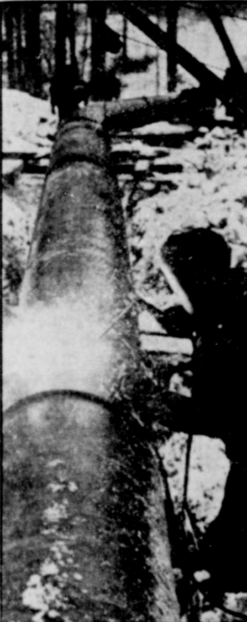
"Big Inch," the world's largest pipeline, pushes through Pennsylvania hill country despite bad weather. Shaped to conform to contour of the hilly ground, the giant pipe rests on skids while welders tack it together. The 1388-mile pipeline will carry oil from Texas to the eastern seaboard.
