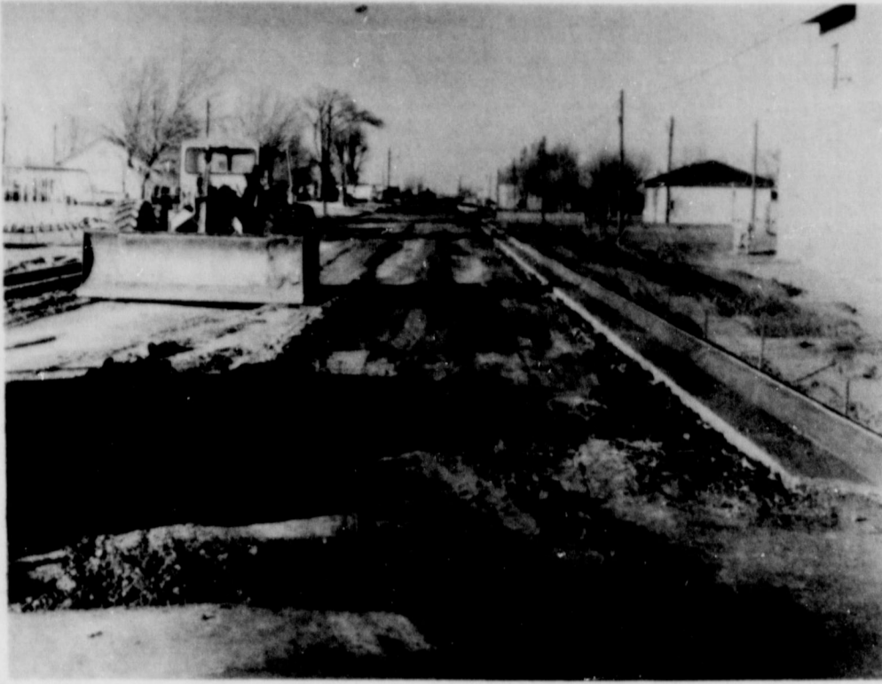
PAVING UNDERWAY. . . Work is currently underway to pave the block on Cleveland Avenue, west of the Junior High Building. When completed, this will take care of what has been a muddy street in wet weather.
