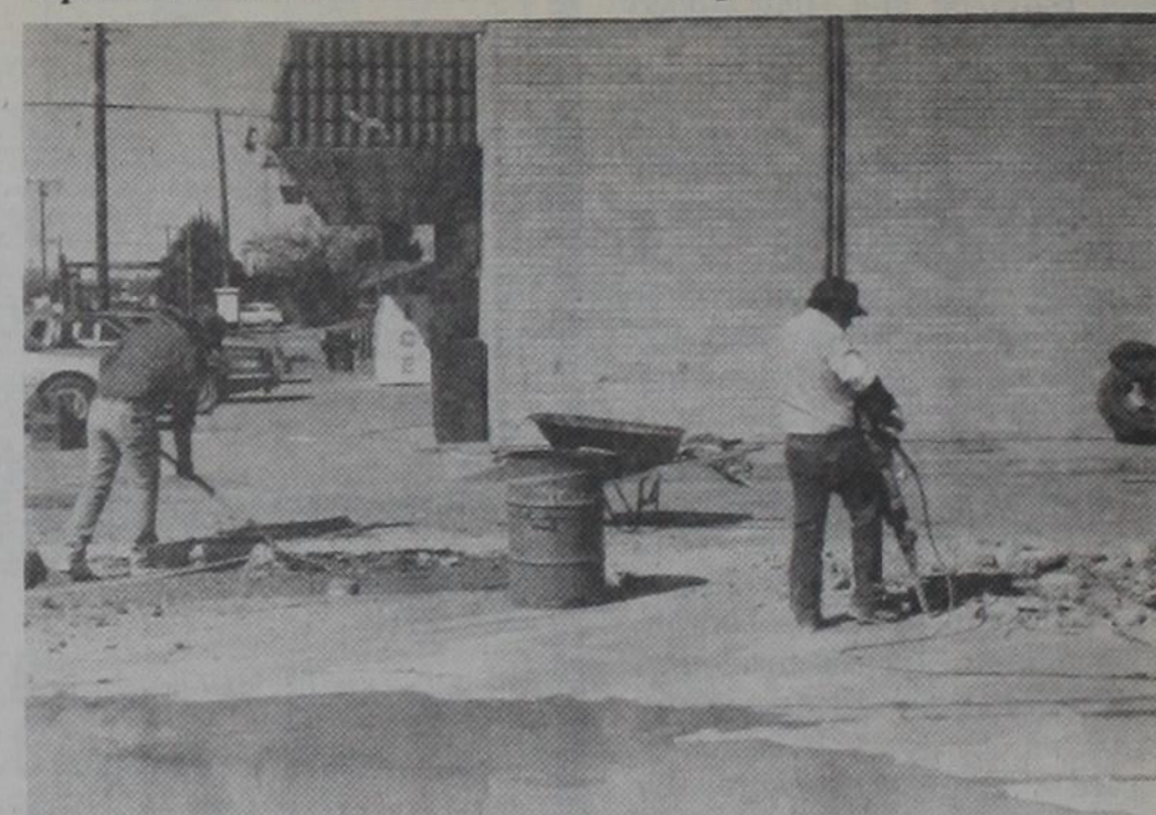
PARKING LOT WORK....Workmen are shown reworking a section of the concrete sidewalk at Allsup's 217 on East Highway 60. Cottrell Construction of Hobbs has been working on the parking areas of both Allsup's stores in recent weeks.
