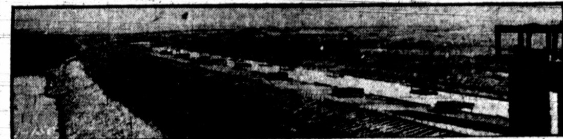
The main storage dam embankment is climbing steadily, with the big dredge piling up its quota of dirt day and night. The top of the completed dam will be about level with the floor of the gate house at the extreme right of the picture.
