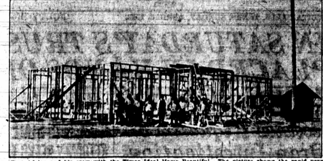
Bert Adria and his crew with the Times Ideal Home Beautiful. The picture shows the rapid progress made in the building of the home since last week when the foundation was laid. Mr. Adria and his crew of expert workmen are putting their very best into this job.
