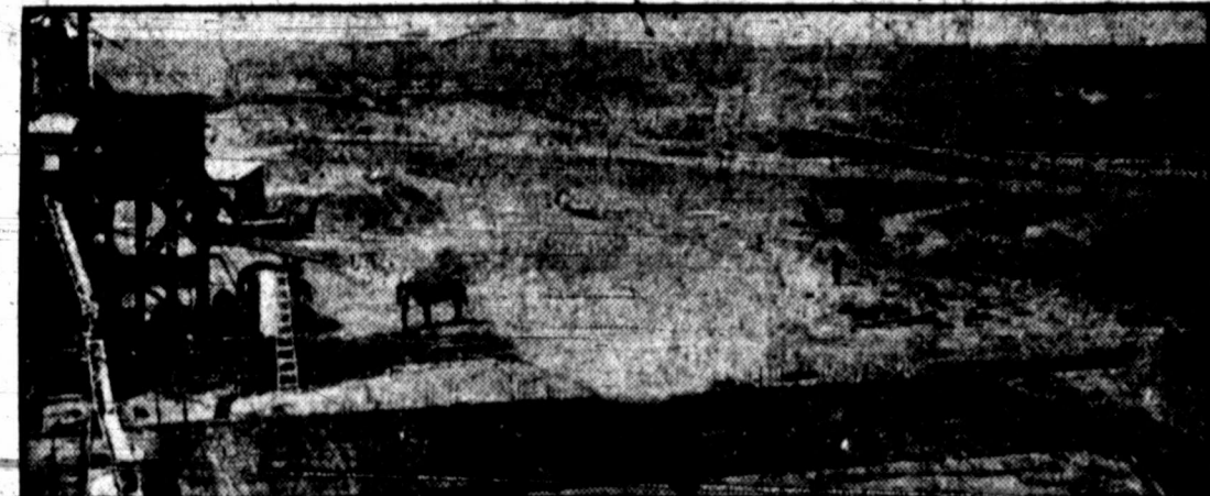
Setting the steel for the floor of the canal head-gate at the diversion dam on which concrete is now being poured.
