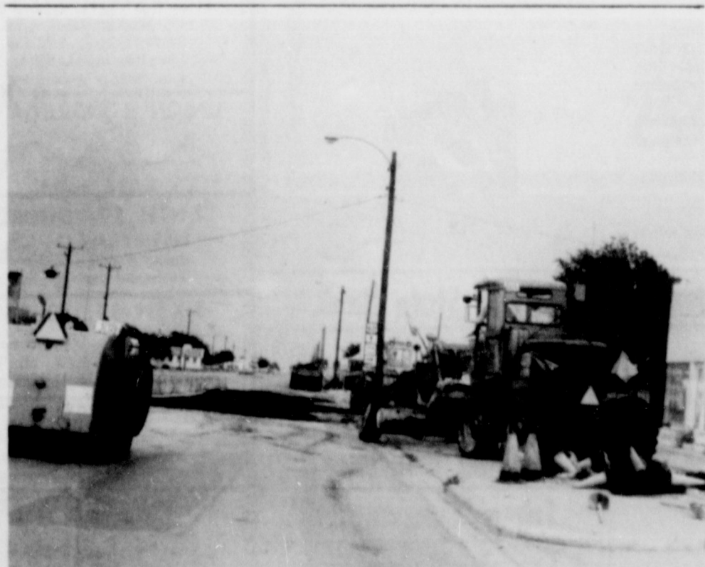
HIGHWAY WORK. . . A construction crew was busy in Friona at the Main Street-Highway 60 intersection, making repairs at the intersection. Traffic was routed around the construction.
