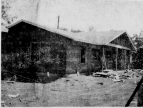
Pictured above is one of the dwellings, located on North Girard St., which is nearer to completion. Roofing has been completed, and it has the look of a real home. As work continues, outside brick and interior work will be added.
