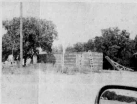
This is the Management Community Building, located on East 4th & Chestnut Streets. When completed, it will cover 1608 square feet of floor space. The building will be complete with kitchen facilities, assembly rooms, lobby and office areas. It will be used for various meetings, reunions, and organizations. Rules and regulations will be set for those who choose to use the building for meetings, etc. It will be constructed of brick and glass, and certainly needed in our town.
