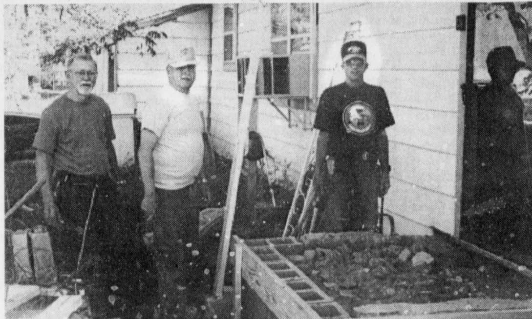
BUILDING A NEW PORCH —Volunteers, Bob Pipes (from left), John Swift and Robert Bennett, start on the project at hand. (Helping Hearts and Hands Photos Courtesy of Wallace Bennett.)
