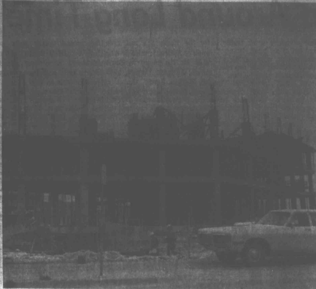
BANK BUILDING GOING UP — Workmen are wasting no time in putting up the new 14-floor Midland National Bank Building bounded by Texas, Illinois, Carrizo and Marienfeld streets. The building is one of many under construction in the Tall City.
