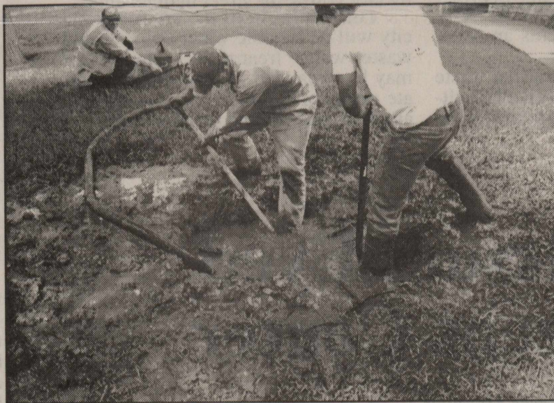
City workers hand dig to find the source of a leak on the Sutton County Courthouse lawn Monday afternoon. The water line is, according to County Judge Carls Garner, supposed to be uncharged. It had previously burst creating havoc at the courthouse.
