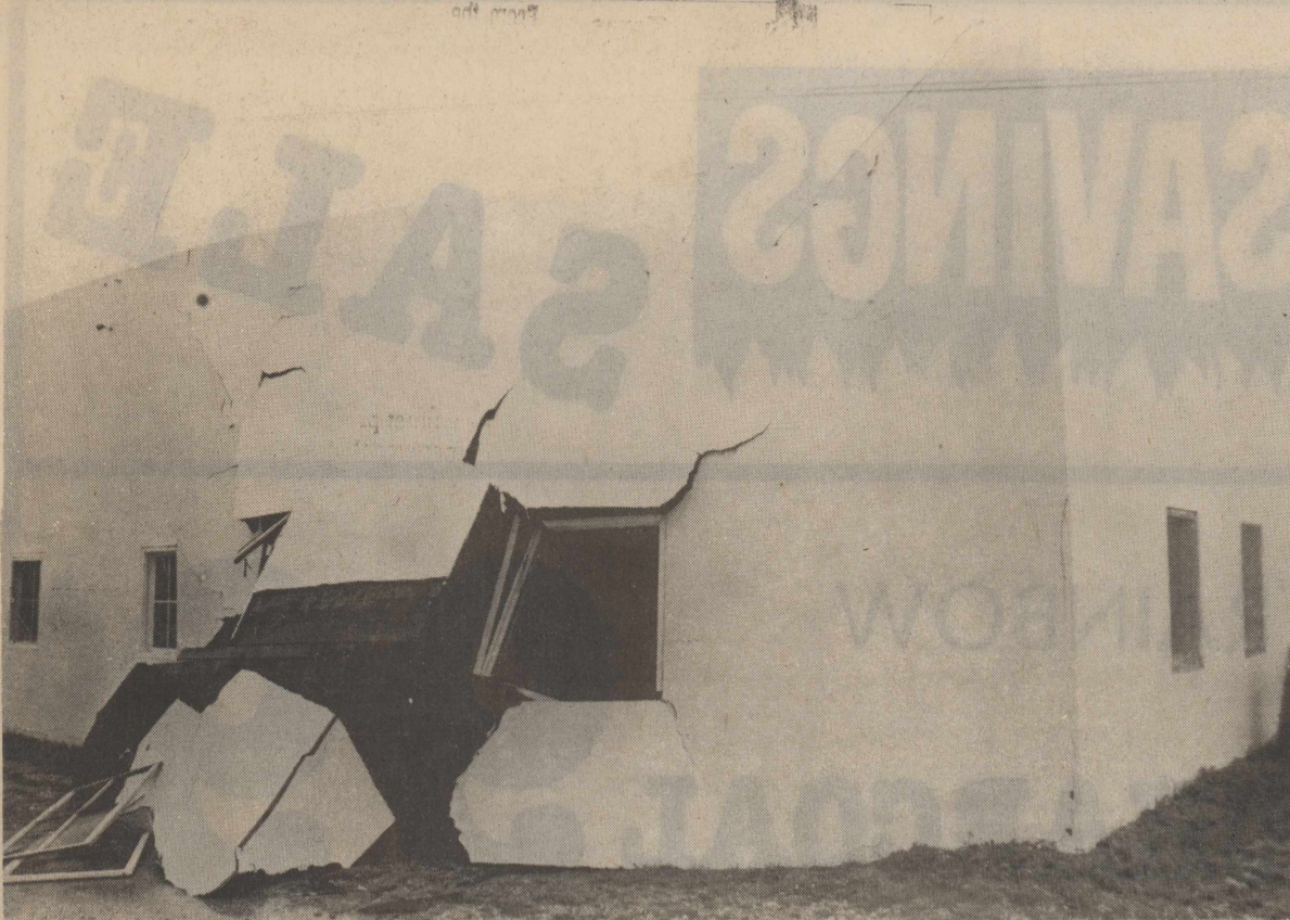
The Talaffero building at the corner of Ave. G and 11th Street lost part of its roof.
