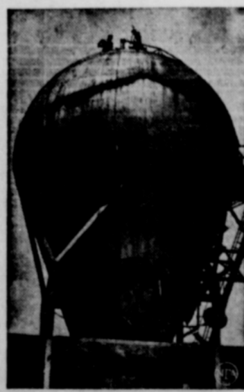
Silhouetted against the clouds, two workmen are dwarfed by the 65-foot Westinghouse atom-smasher in Pittsburgh, Pa., as they resurface the giant tank to prepare it for a research program aimed at harnessing atomic power for peacetime use.
