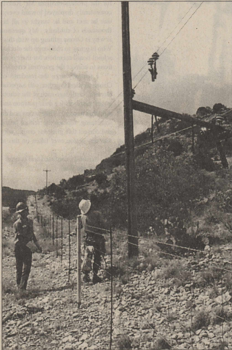
RIO GRANDE ELECTRIC CO-OP employees Joel Duarte and Stephen Ramirez, of Fort Stockton survey the damage to a high voltage pole on the Bill Clegg Ranch on the South Pandale Road Monday morning. Arcing high voltage caused by dust collecting on the pole caught the pole on fire. Ozona Volunteer Fire Department firemen quickly extinguished the flames. photo by Scotty Moore
