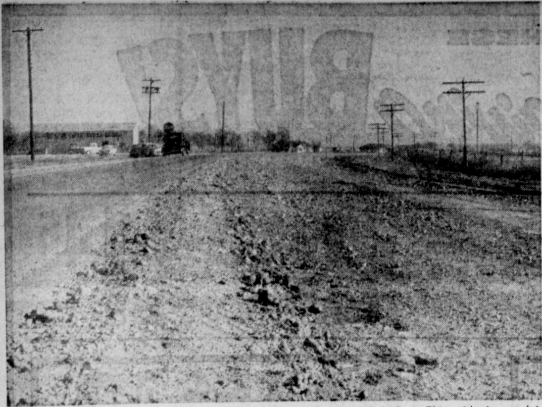
HIGHWAY WIDENING PROJECTS continue to forge ahead in Muleshoe. This widening and improvement of US 70 is being done on the road north of Muleshoe, while preliminary work is going on in town on the widening of 70-84 to the west city limits, and another crew is working on 84 east to the Lamb county line.
