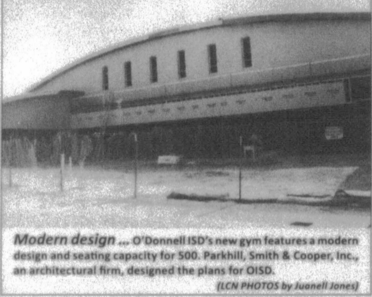
Modern design ... O'Donnell ISD's new gym features a modern design and seating capacity for 500. Parkhill, Smith & Cooper, Inc., an architectural firm, designed the plans for OISD.
