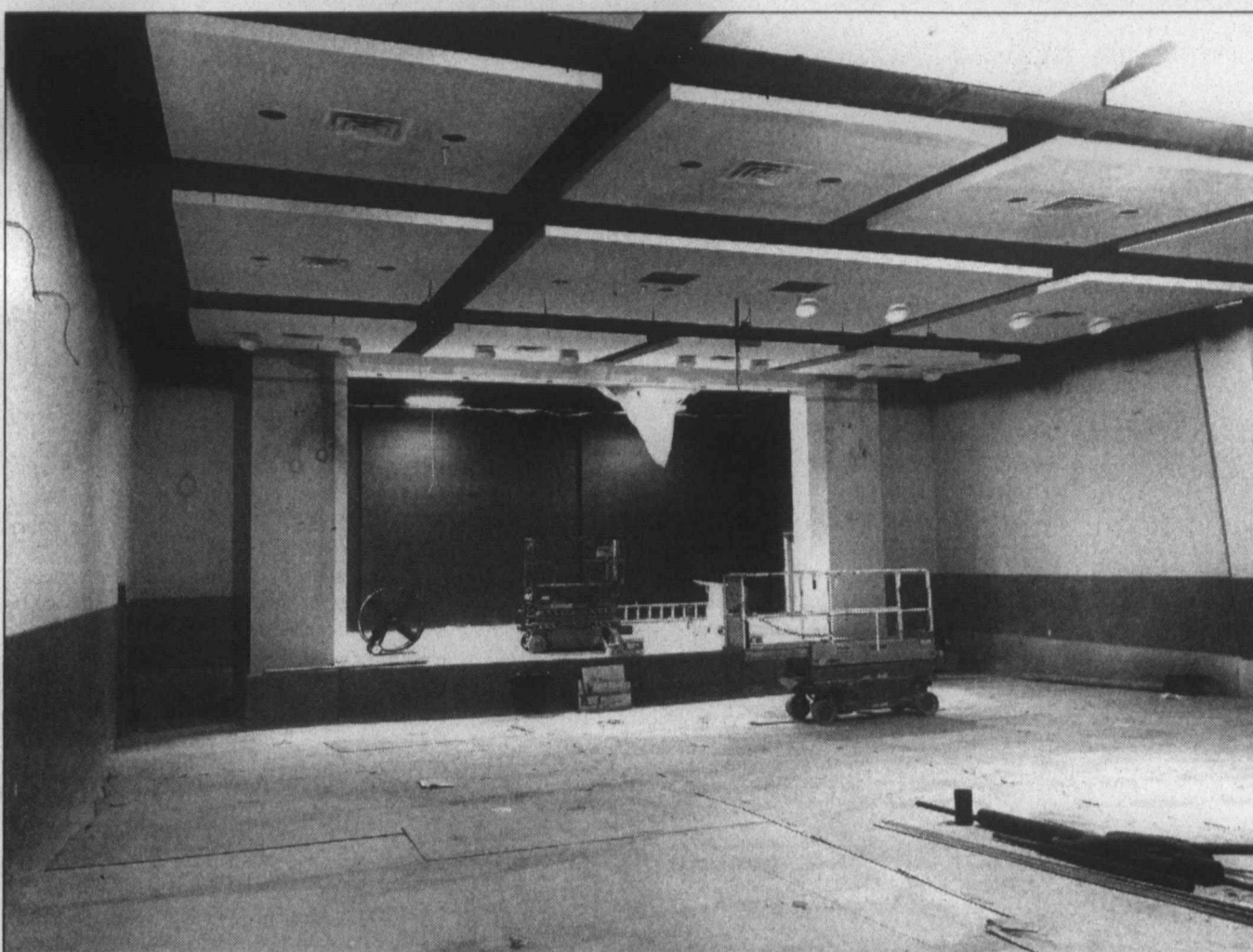
New auditorium ... The Tahoka ISD auditorium is still undergoing construction on the TISD campus. Pictured here is the interior of the new auditorium, with finishing details still needed throughout, as well as flooring and seating, before the building can be used. This week, paving outside the building was continuing. (LCN PHOTO by Juanell Jones)
