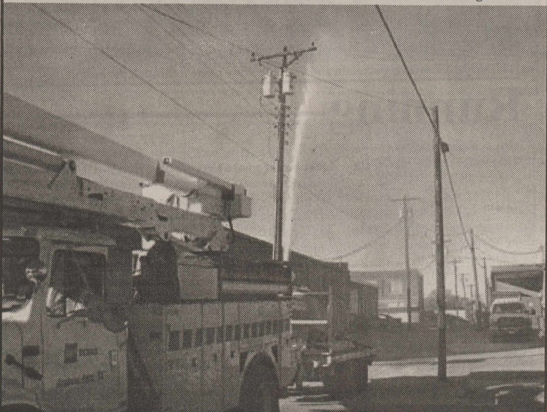
WASHING OFF TRANSMITTERS —AEP sprayed the transmitters to clean off soot and smoke. (Photo courtesy of Vanda Anderson)
