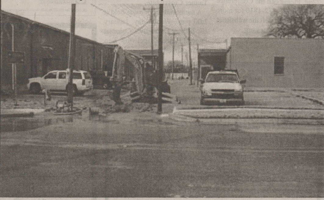
CITY AND DAL-MAR EMPLOYEES WORKING HARD Severe temperatures busted a line between Higginbotham's and the Post Office.
