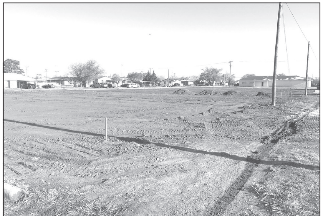
Work has begun on the new housing project at 6th and Ashland. Phase 1 calls for the building of one (1) triplex residential property and one (1) quadplex residential property on Lots 10-12. Completion date for Phase 1 is scheduled for the end of October 2020. Stay tuned.
