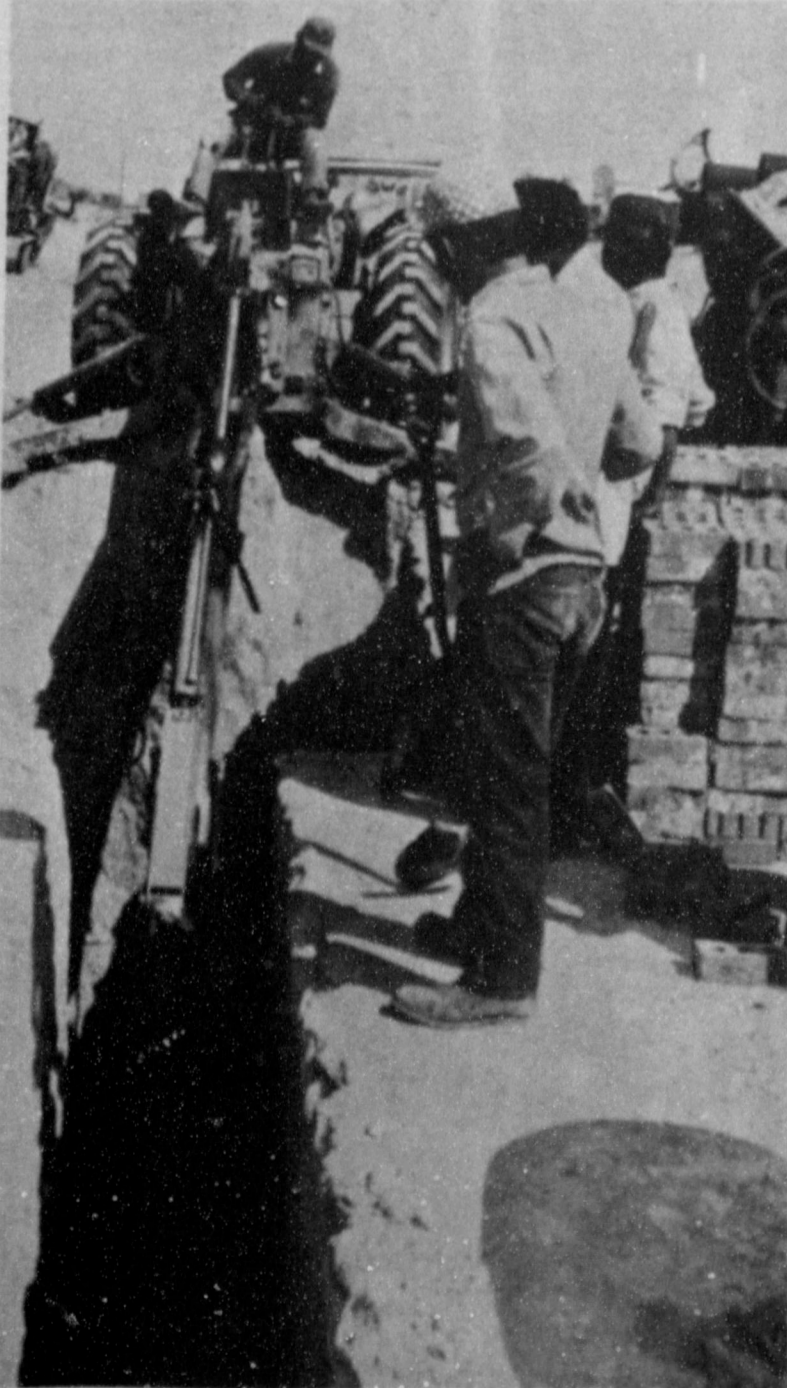
DOWN GO THE SEWER LINES .....Vaughn Construction Company is busy laying sewer lines to the Country Club addition, which was recently annexed into the Muleshoe City limits.
