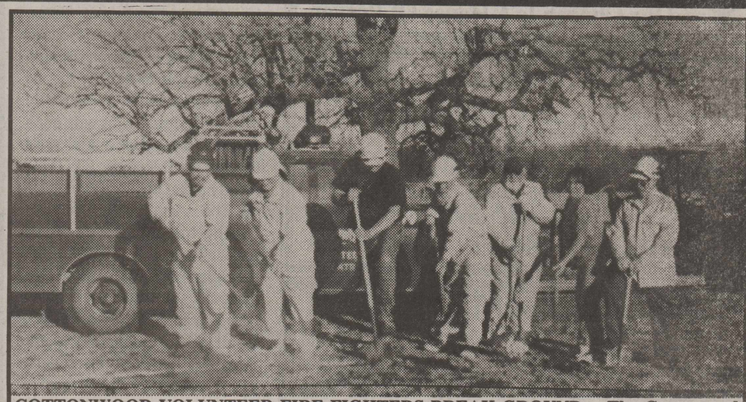
COTTONWOOD VOLUNTEER FIRE FIGHTERS BREAK GROUND— The Cottonwood Volunteer Fire Control Unit celebrated with a ground breaking celebration March 16, 2009. Pictured from left to right are Joe Terstege, Roger Hinkle, Annie Smith, Ken Farmer, Buel Neff, Norma Farmer and Tom Bennett.
