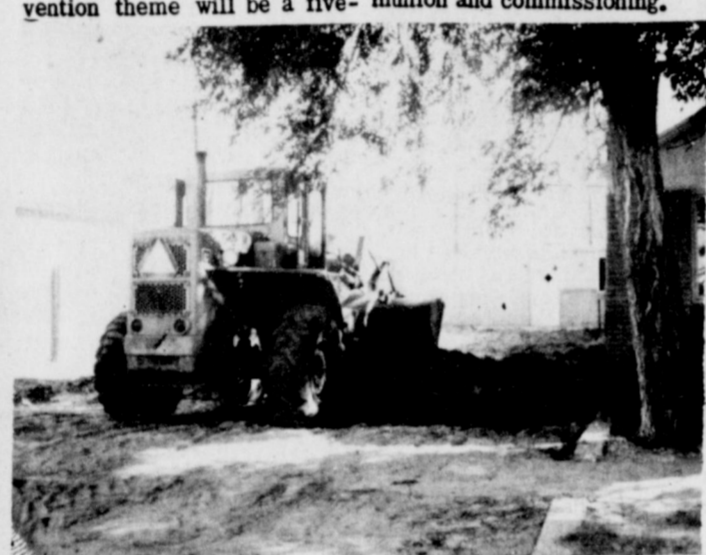
NEW PATIO . . . Work began this week on a new patio for the Muleshoe Nursing Home. The patio and future garden spot is being done through donations of money and labor.
