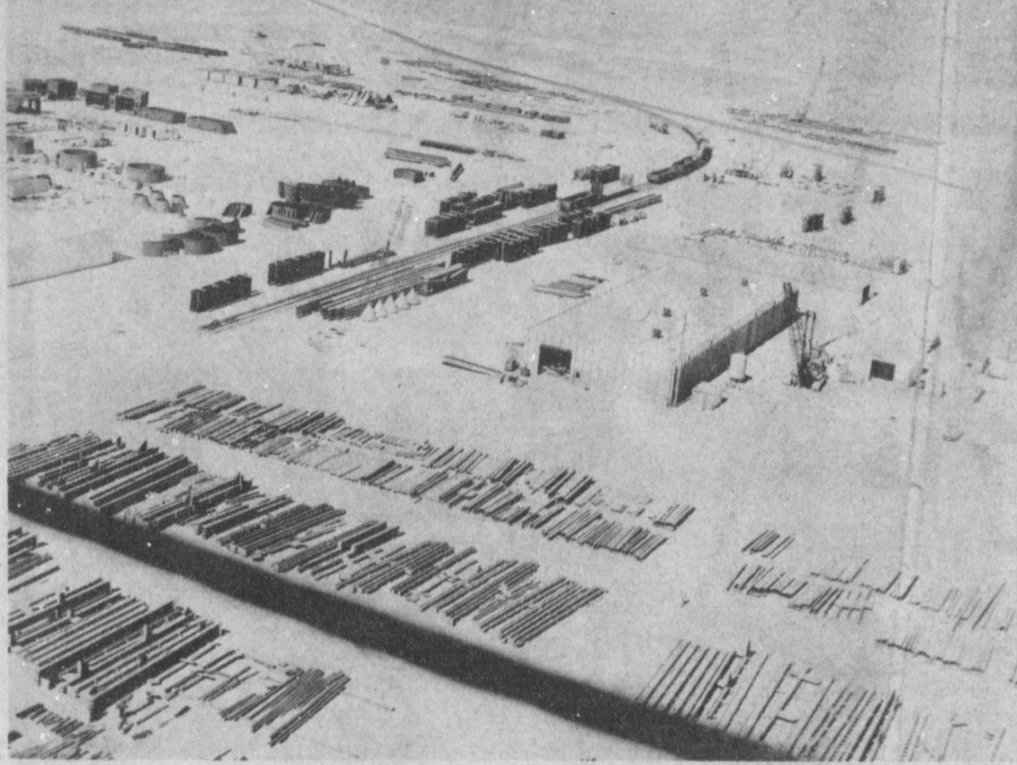
TOY RAILROAD SERVES TOLK CONSTRUCTION SITE.... Appearing to be a toy train on the track is the background of this picture. A spur from the main line of Santa Fe Railway was run to the Tolk Station Construction site near Muleshoe. The steel in the foreground was brought in on the train to unload. Asouthwestern Public Service Co. official, Bob DeLoach, said the trains bypass the spur, then back in to the site as the turnaround has not been completed yet. After unloading, the trains go straight back to the main line.
