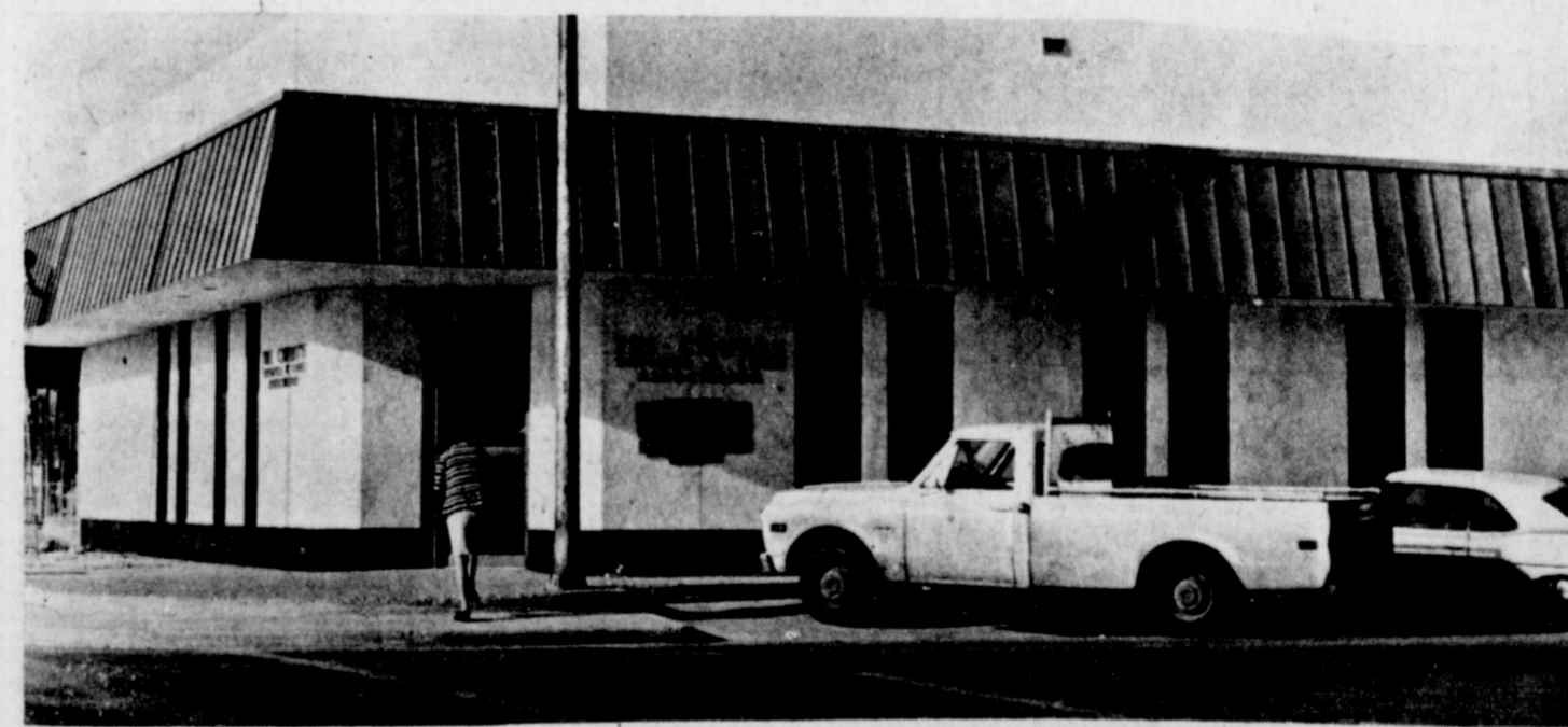
CONSTRUCTION CONTINUES . . . Construction on the new home of Tri-County Savings and Loan Association in Muleshoe continues. The marble walls have been erected and work on the out-
