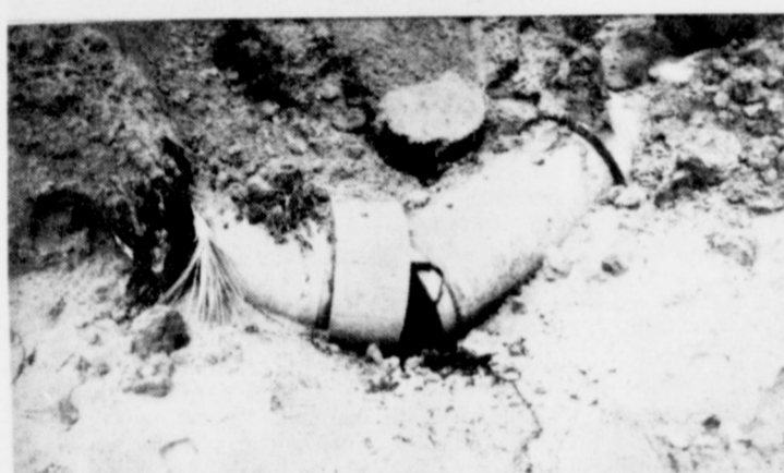
WATER TANK COLLAPSES . . . The southeast side (top) of the one million gallon round storage reservoir collapsed over the weekend, breaking out a piece of concrete 20 feet long and up to four feet in width out of the tank floor. It washed out a gully 30 feet across the top, about 15 feet deep. (Middle) A feeder line, one of the four water wells that feed the tank, was also broken apart. (Bottom) The lower picture is of concrete section of a line of AC pipe that feeds the tank, as it was damaged by the million gallons of water that rushed out when the floor gave away.
