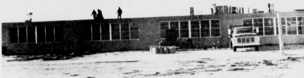
JUNIOR HIGH ROOF DAMAGED . . . Damaging winds that hit Muleshoe Saturday did considerable damage to the roof of the Muleshoe Junior High School as well as the gym. Workmen were busy early Monday morning starting repairs.
