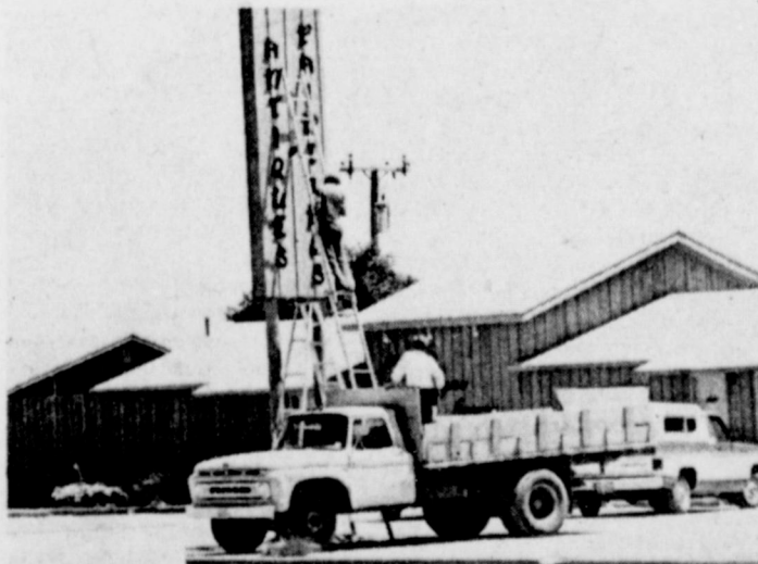
NEW SIGN... Workmen are placing a new sign at the large complex housing the Art Loft on West American Boulevard. The unusual sign was added to complement the art, painting and antique center.
